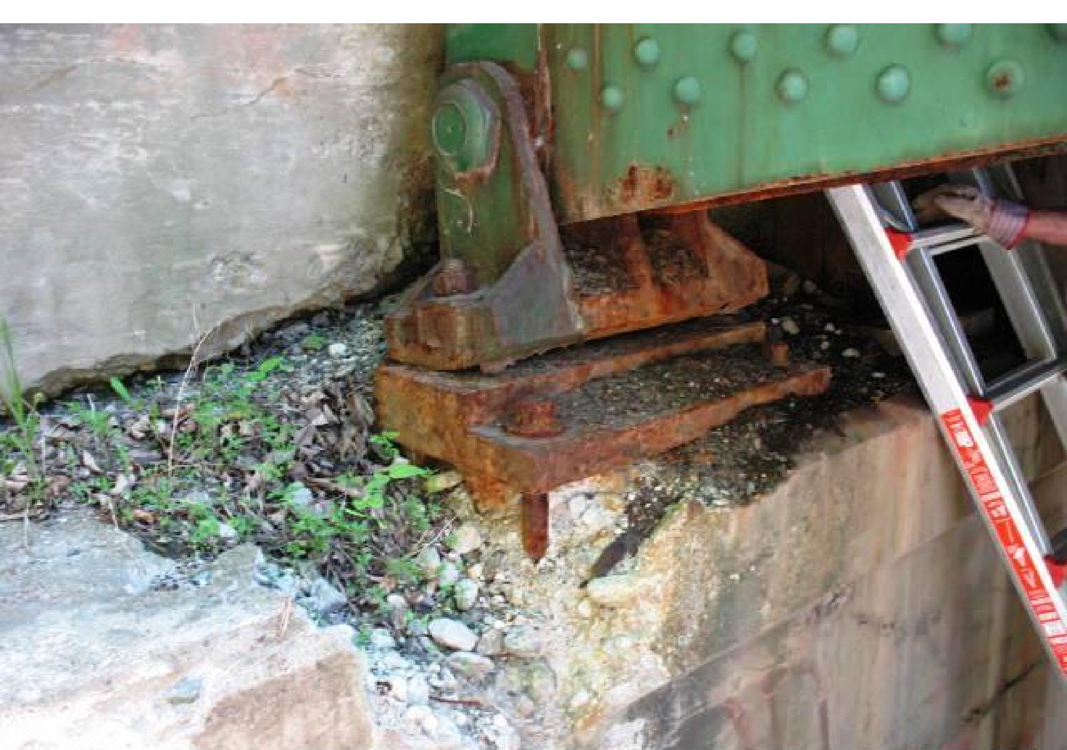
Undermining of the over rotated bearing support.
