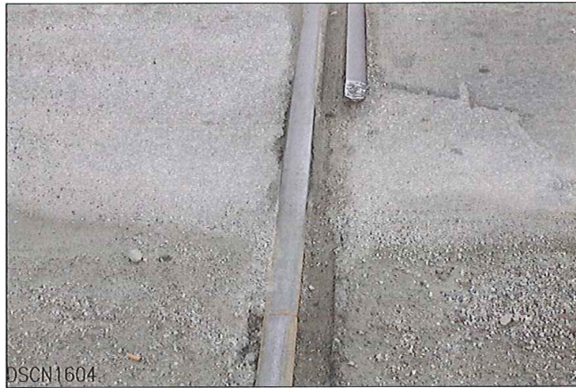
BROKEN MUDRAIL - NORTH RAIL
