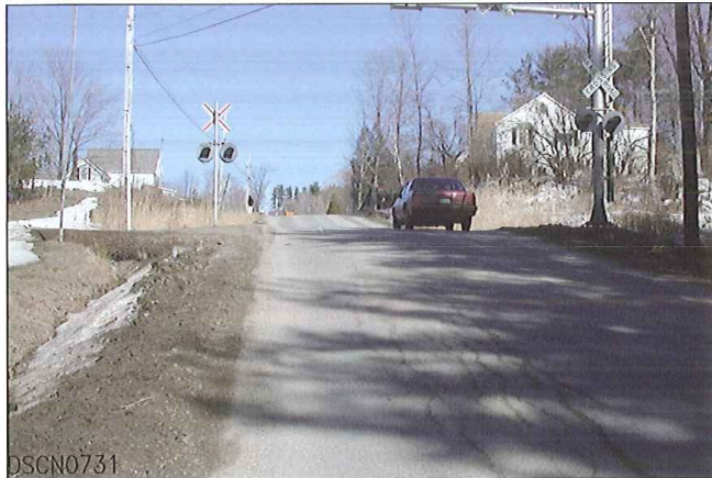
LOOKING FROM SOUTH TO NORTH SHARP GRADE BREAK
