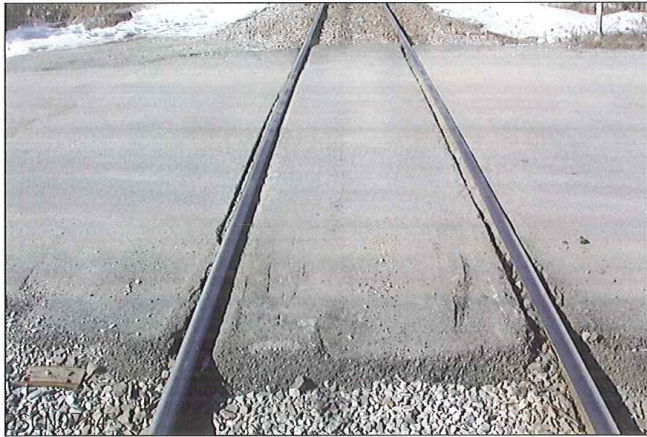
LOOKING FROM EAST TO WEST NO MUDRAIL INSTALLED
