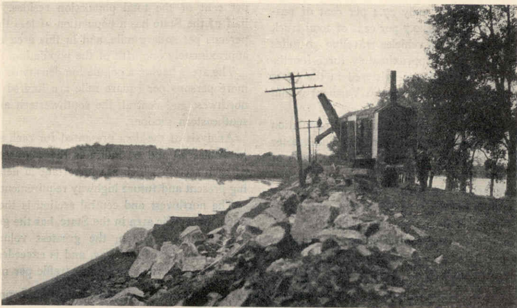
Placing riprap on the Sand Bar highway, between South Hero and Nutton
