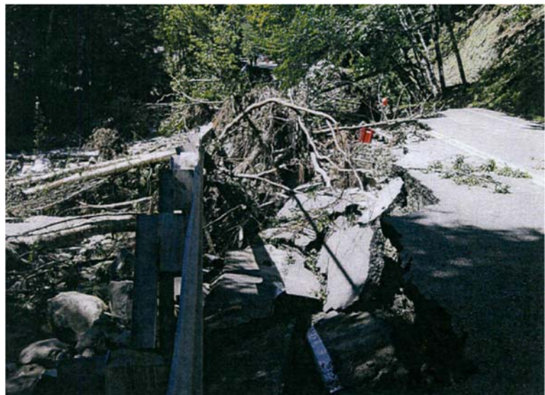
Figure 2 - Erosion damage of Vermont Route 9 during Tropical Storm Irene at the Marlboro-Brattleboro. Photo Source: VTrans
