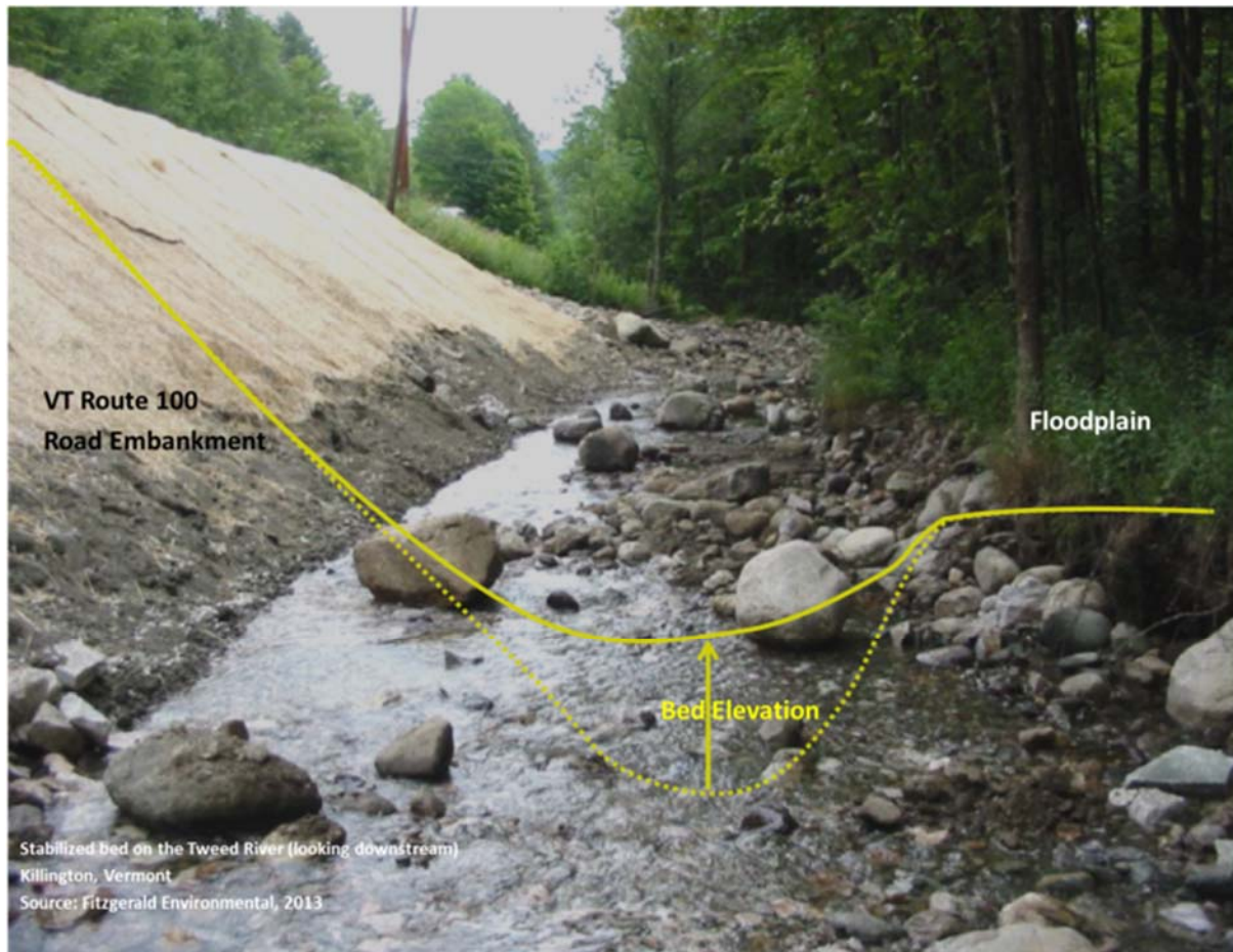
Figure 8: Elevated channel via bed armoring right after construction. Note the reconnected floodplain and the gentler side slope of the road embankment. (Source: Fitzgerald Environmental, 2013)
