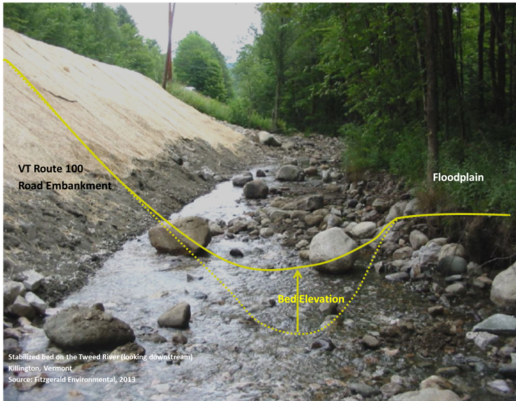
Figure 20 Elevated channel via bed armoring right after construction. Note the reconnected floodplain and the gentler side slope of the road embankment. (Source: Fitzgerald Environmental, 2013)
