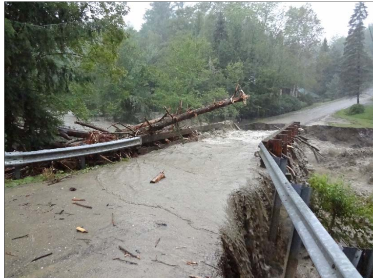
Figure 2 - Significant damage during Tropical Storm Irene, Town of Stockbridge. Photo Source: David Brown, Road Foreman
