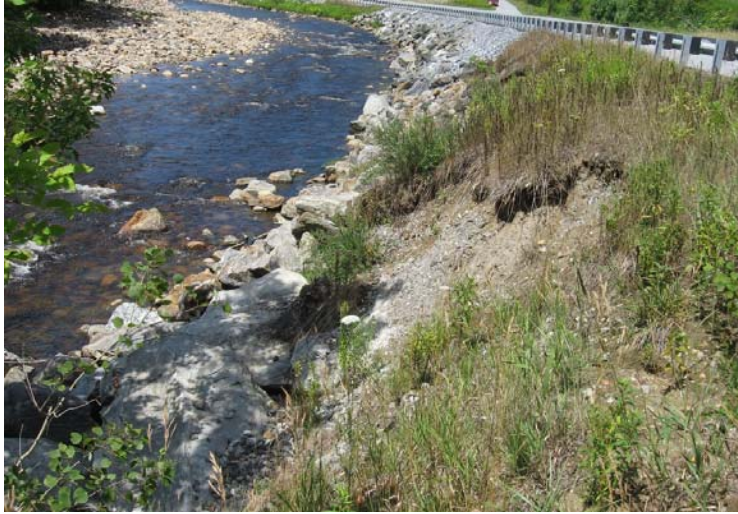
Figure 6: Erosion along Vermont Route 9 following emergency repairs after Tropical Storm Irene. (Source: R. Schiff, 2012).
