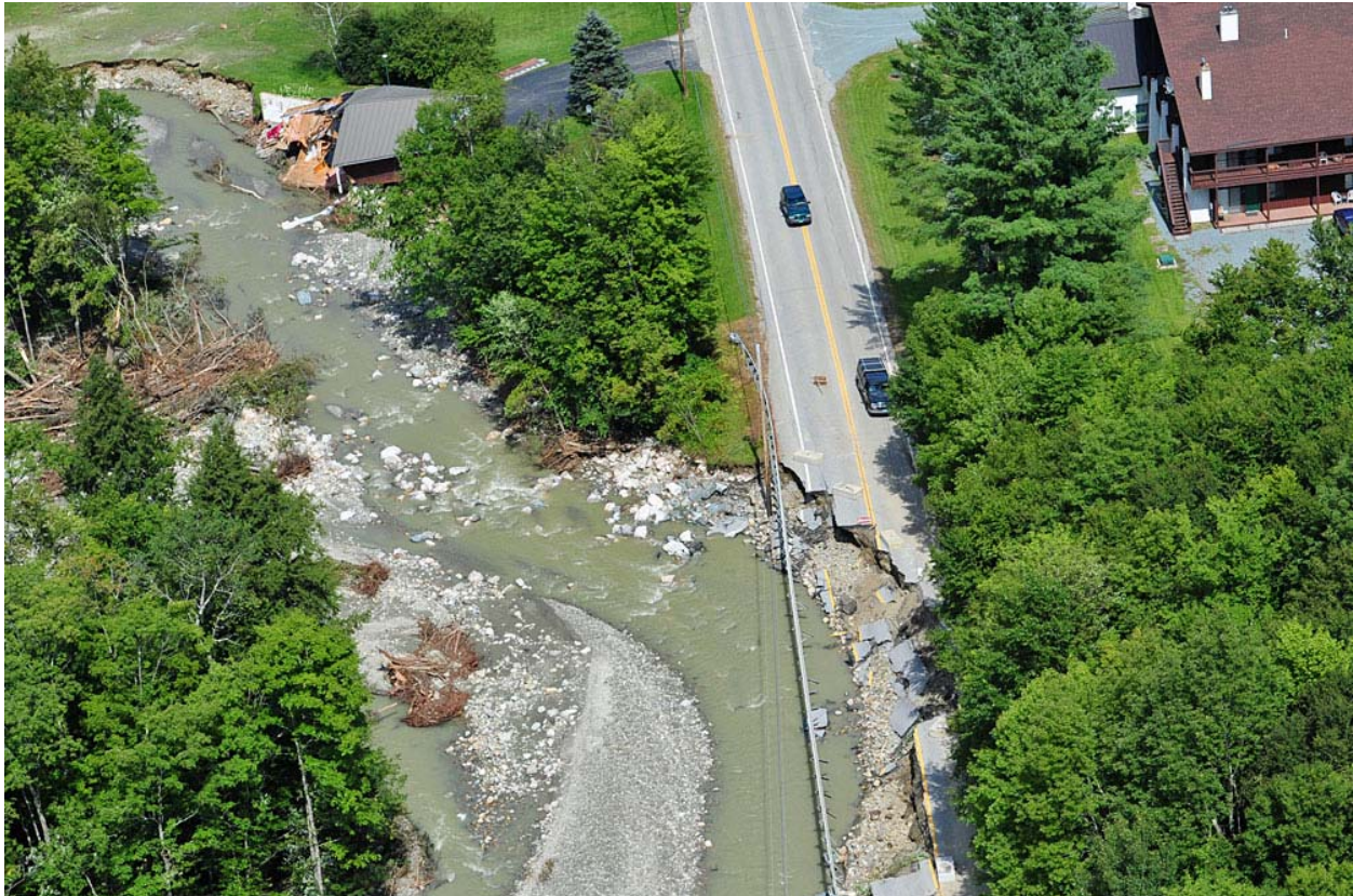
Figure 5: Failure of the Vermont Route 100 road embankment due to erosion during Tropical Storm Irene in Pittsfield. (Source: Mansfield Heliflight, 2011)
