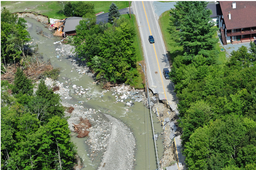
Figure 17 Failure of the Vermont Route 100 road embankment due to erosion during Tropical Storm Irene in Pittsfield (Source: Mansfield Heliflight, 2011)
