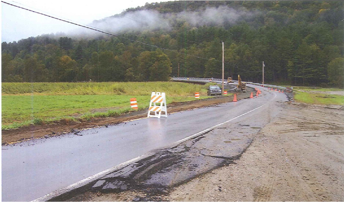
Figure 9: Road repairs following inundation and deposition damages during Tropical Storm Irene. (Source: VTrans, 2011)
