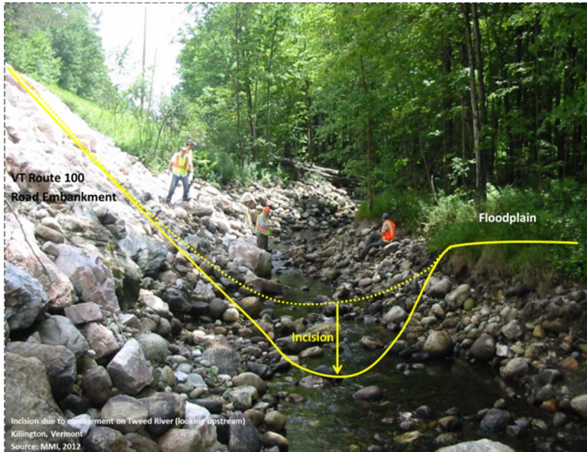
Figure 7: Incision and floodplain disconnection due to confinement on Tweed River following Tropical Storm Irene in Killington, Vermont. (Source: MMI, 2012)
