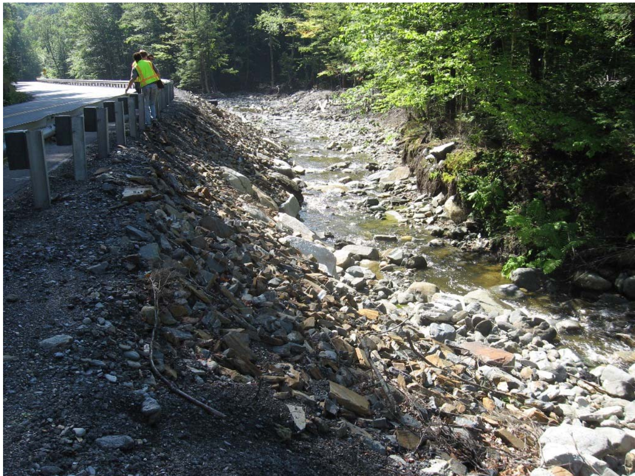
Figure 9: A pinch-point in the channel where the Vermont Route 9 embankment was eroded during Tropical Storm Irene. (Source: MMI, 2011)
